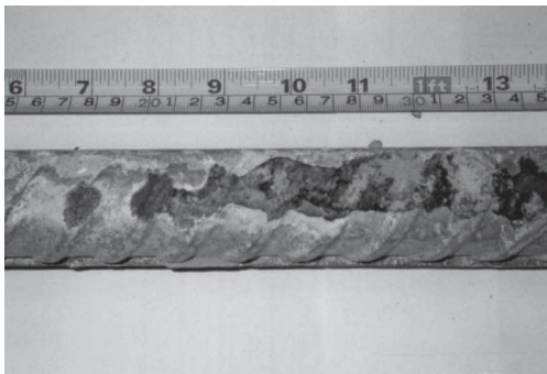
Plate 3 – Rusting of Zinc Coating and Steel Reinforcement
