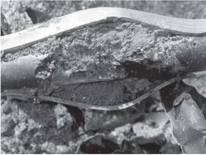
Plate 1 – An Exhumed Soil Nail Showing Soil Trapped between Steel Bar and Centraliser
